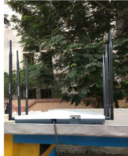
Router 3 is wirelessly bridged to Router 2 and provides internet access to the users
